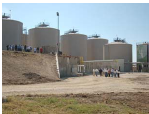
Figure 11: Microgy Inc biogas production and conditioning facility in Texas. source: Microgy Inc.
